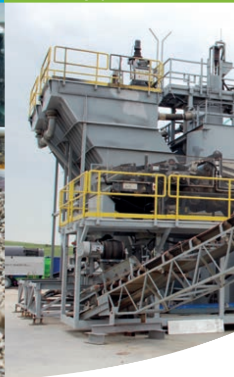
Thermal desorption soil cleaning system
