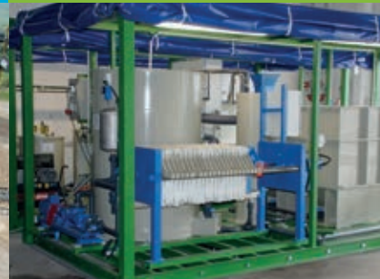
Mobile wastewater treatment unit
