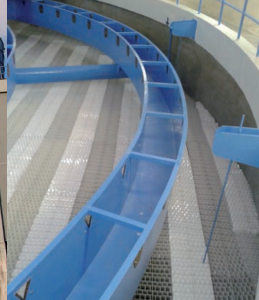
Tube settling modules in drinking water pretreatment
