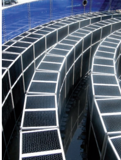
Fixed bed media in industrial waste water treatment
