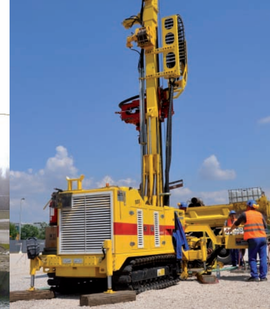
Pumping and monitoring wells
