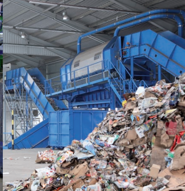
Communal waste processing plant
