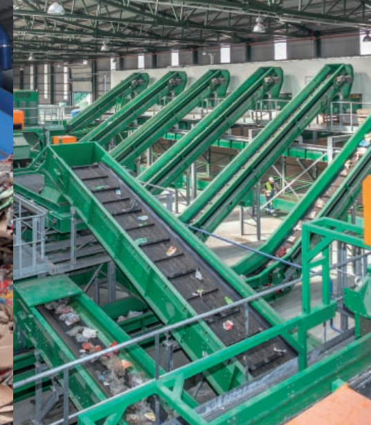
Communal waste processing plant
